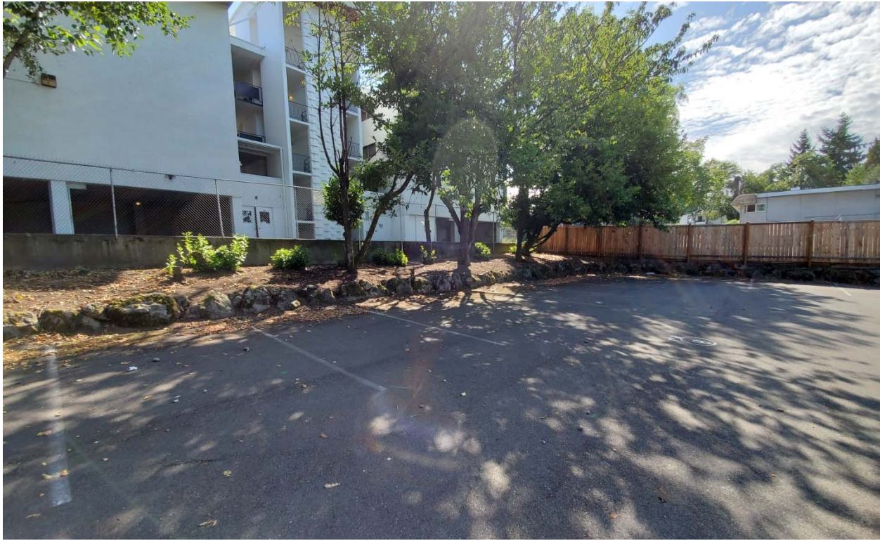
Photo 2: CIP wall and rockery along the southern perimeter of the site, looking southwest.
