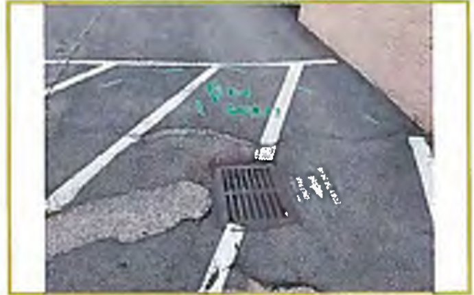
Photograph #26: Stormwater 'dry well', located outside driveway for hearse, basement level.
