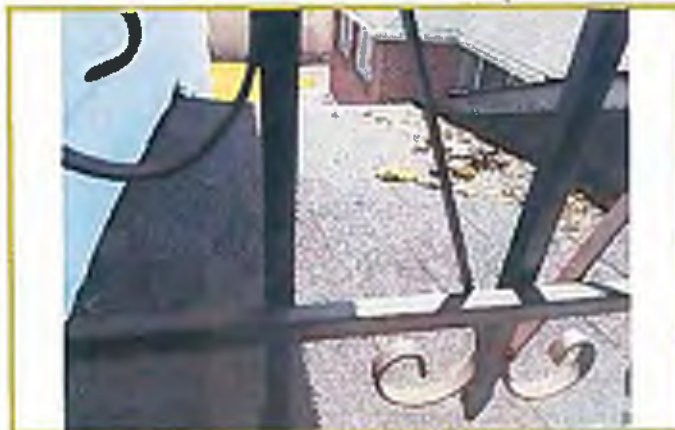
Photograph #33: View from attic window of funeral home manager's residence, showing asphalt shingle roofing material.
