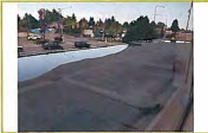
Photograph #25: View from 2 nd level of funeral home, showing torch down roof. Looking northwest.
