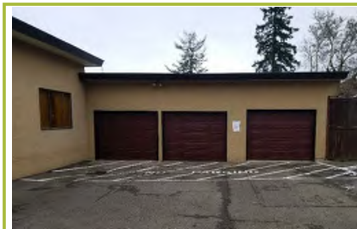
Photograph #24: Garage entry for hearse, located south of funeral home – basement level.
