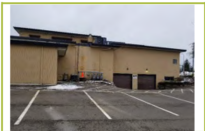
Photograph #27: East exterior wall of the mail funeral home, looking west from rear parking lot.
