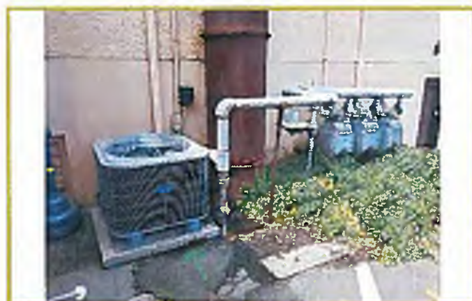
Photograph #16: Natural gas service for crematoria, crematory exhaust stack, and air conditioning unit, located outside east building wall, basement level.
