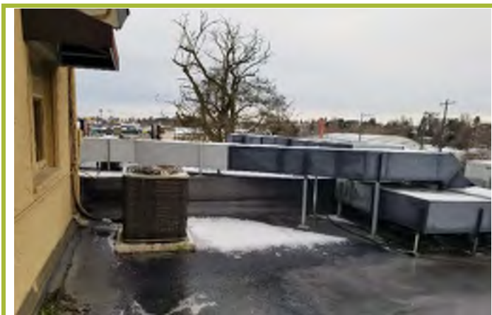
Photograph #23: View from upper level looking at HVAC equipment on roof of main level. Looking north-northeast.
