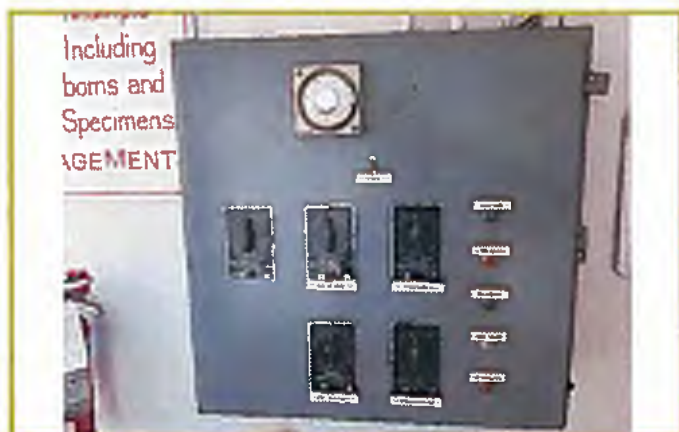
Photograph #15: Crematory controls.
