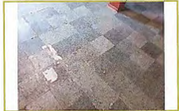
Photograph #34: Basement of funeral home manager's residence, showing tile with apparent water damage Description
