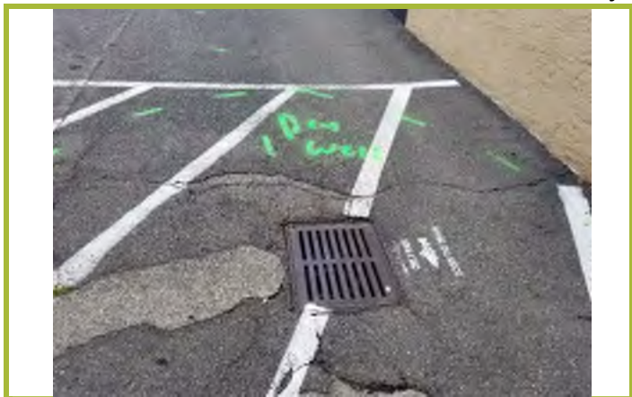
Photograph #25: Stormwater 'dry well', located outside driveway for hearse - basement level.
