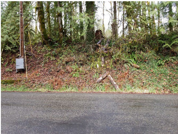
Photo 3. OWS 3 existing pole to be replaced.
