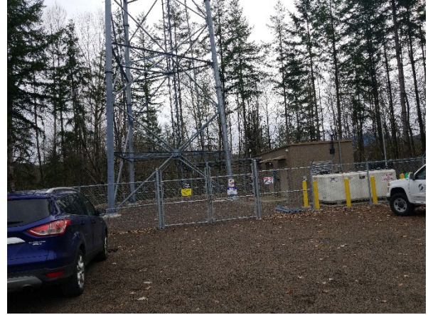
Photo 20. Existing PSERN SWAN antenna site.
