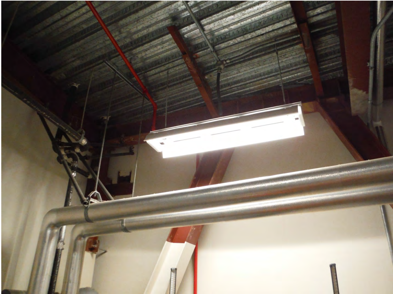
Figure 19. Non-Concentric Braced Frame in WPTP Admin-Operations Building
