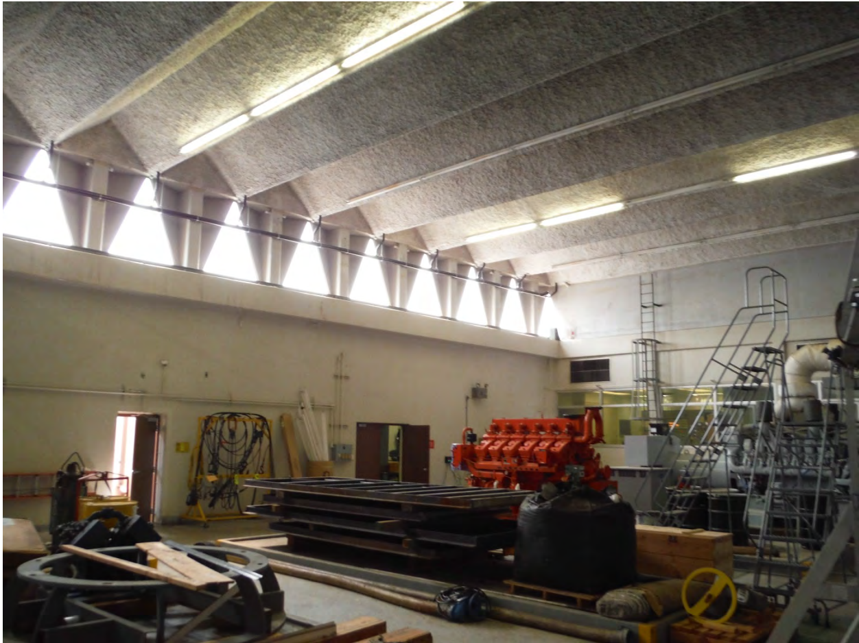
Figure 3. Interior View of Matthews Park Pump Station, Including Interveted-V Roof System and Pre-Cast Concrete Weak Story Framing
