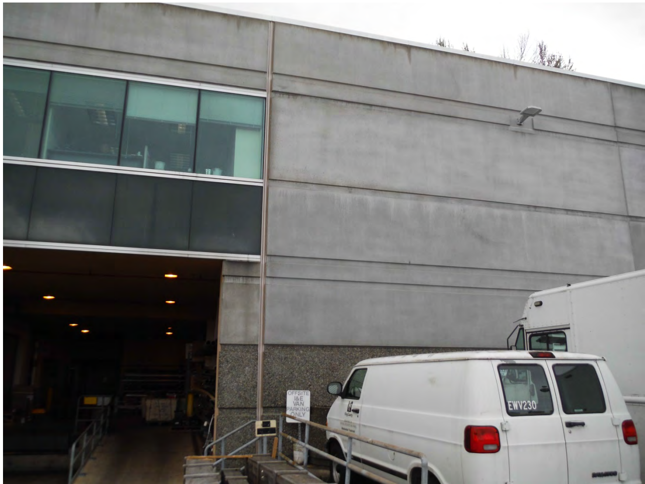
Figure 3. Insufficient Seismic Joint between Adjacent Building
