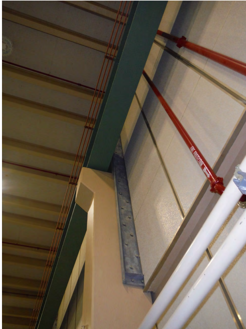
Figure 3. Interior View of STP Effluent Pump Station, Seismic Retrofit to Concrete Column (Extent and Criteria/Objectives of Retrofit Unknown)
