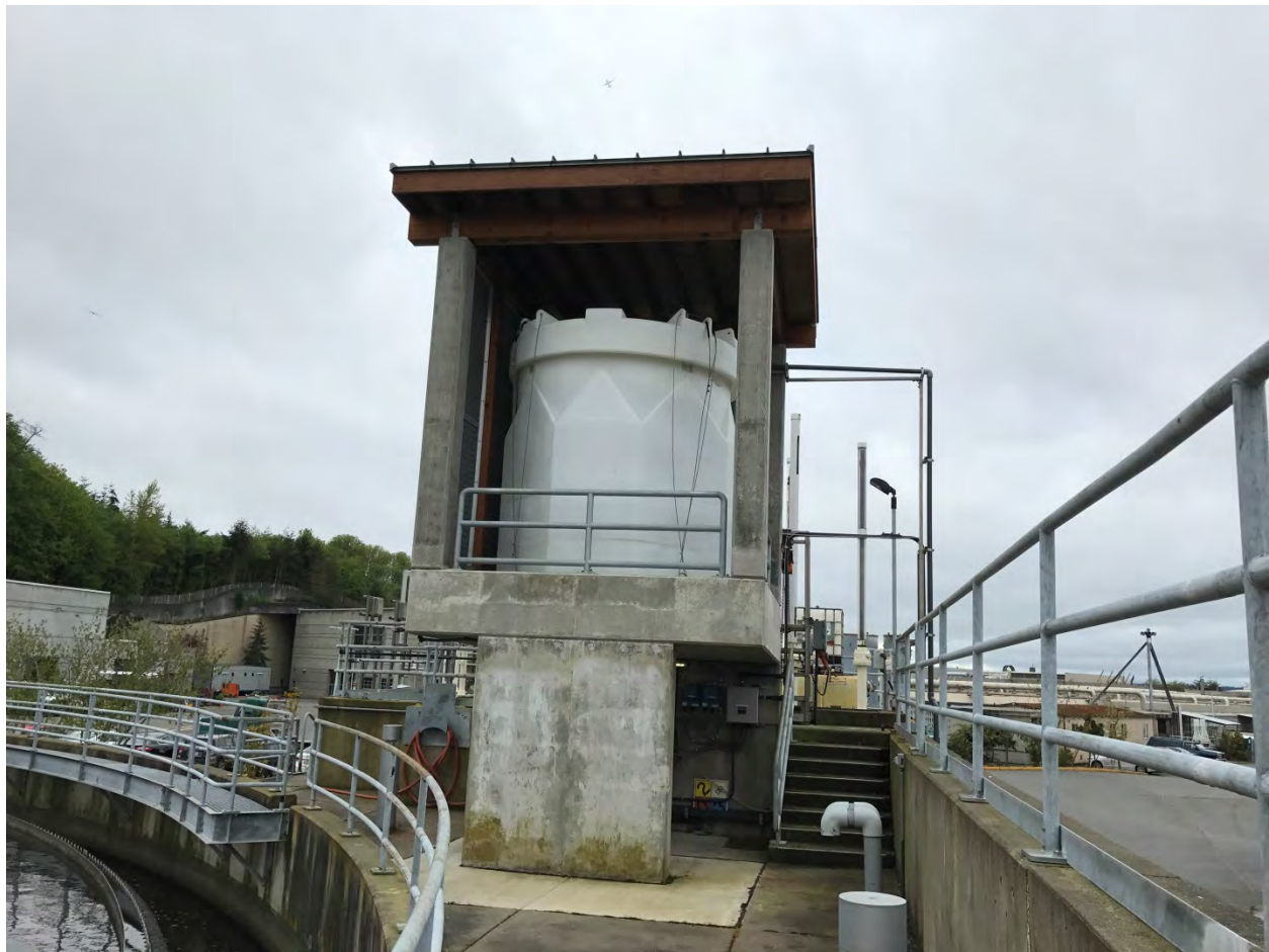
Figure 22. WPTP Hypo Mixing Tank and Support Frame
