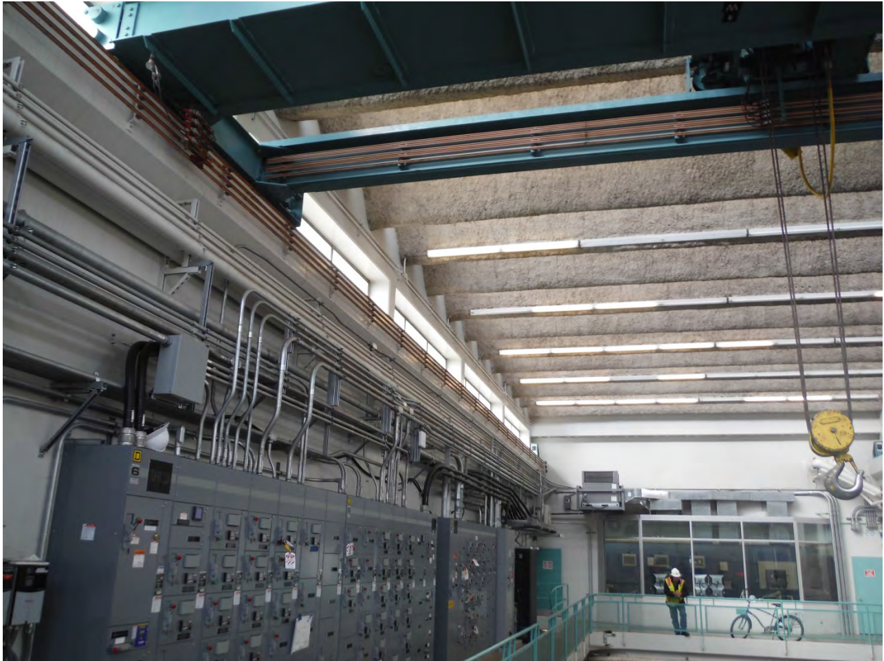
Figure 4. Interior View of Raw Water Pump Station, Including Z-Beams and Weak Story
