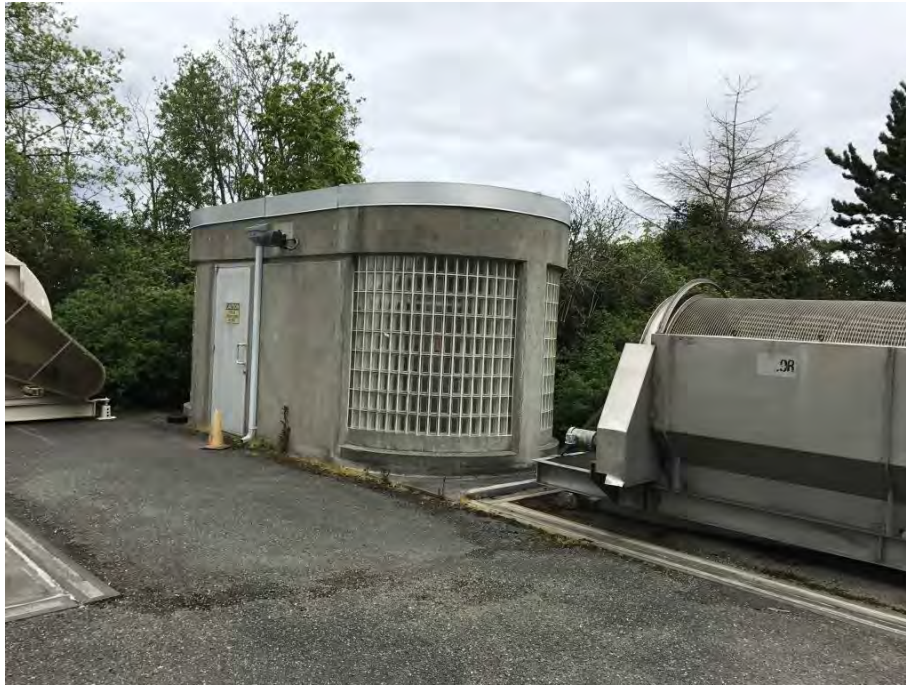
Figure 34. West Point Treatment Plant Intermediate Pump Station Glass Block Walls at Ingress/Egress Stairway Example
