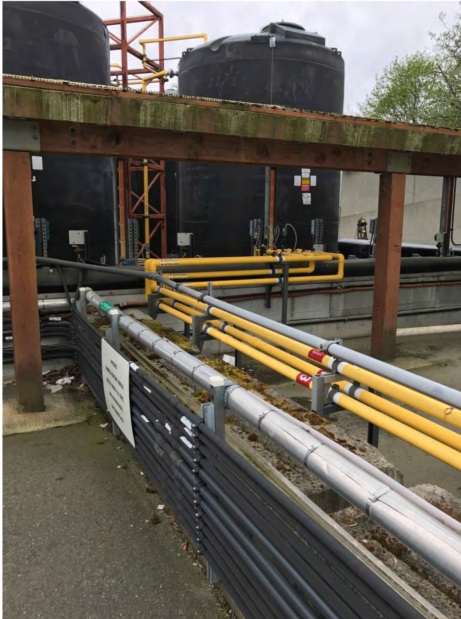
Figure 2. WPTP Hypo Mixing Tanks
