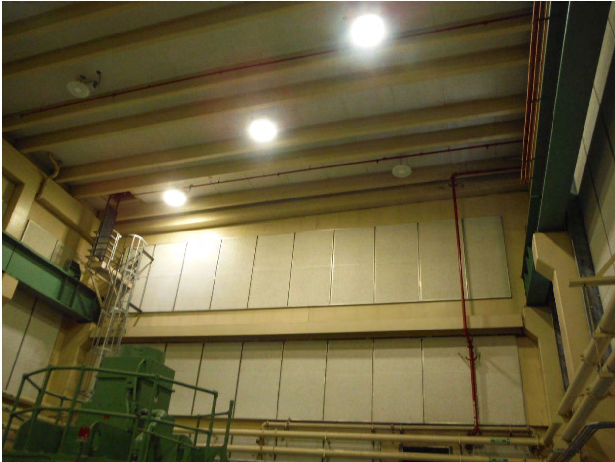
Figure 30. Interior View of STP Effluent Pump Station
