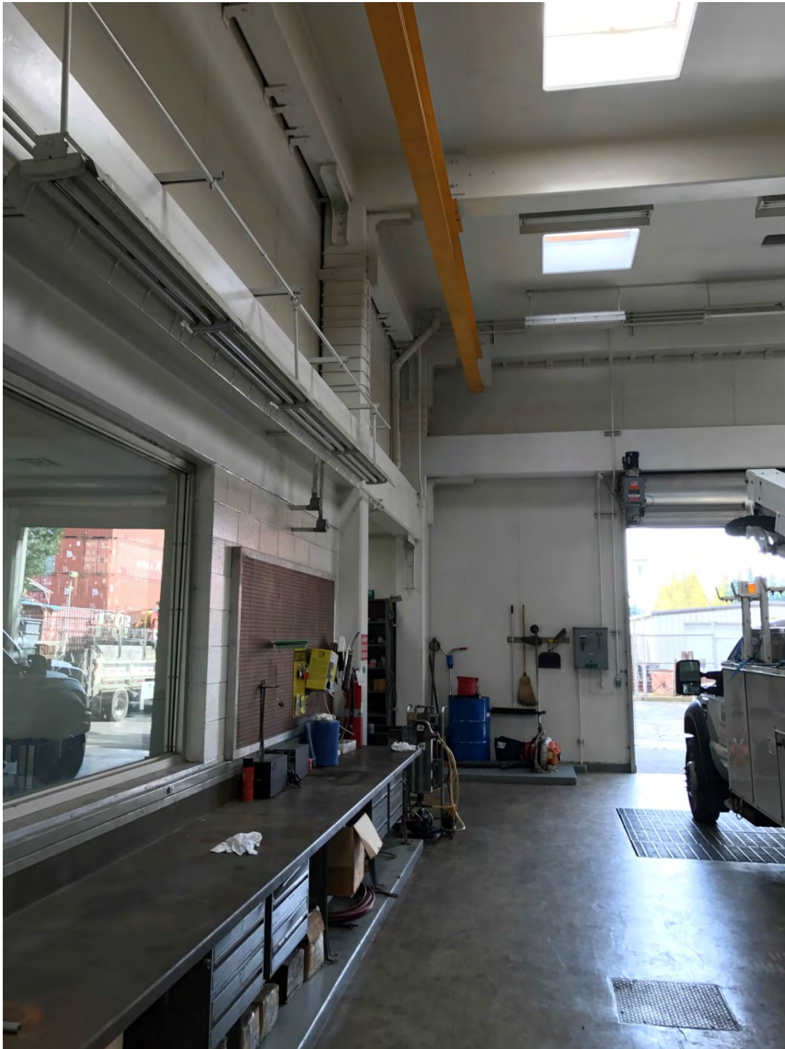
Figure 10. Interior View of Duwamish Pump Station, including Limited “Bolts Plus” Seismic Upgrade of Non-Ductile Moment Frame Column
