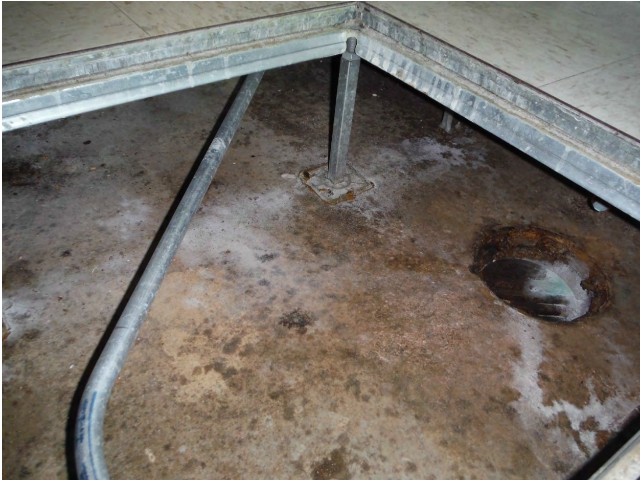
Figure3. Raised Floor Missing Braces/Hold-Downs in WPTP Admin-Operations Building
