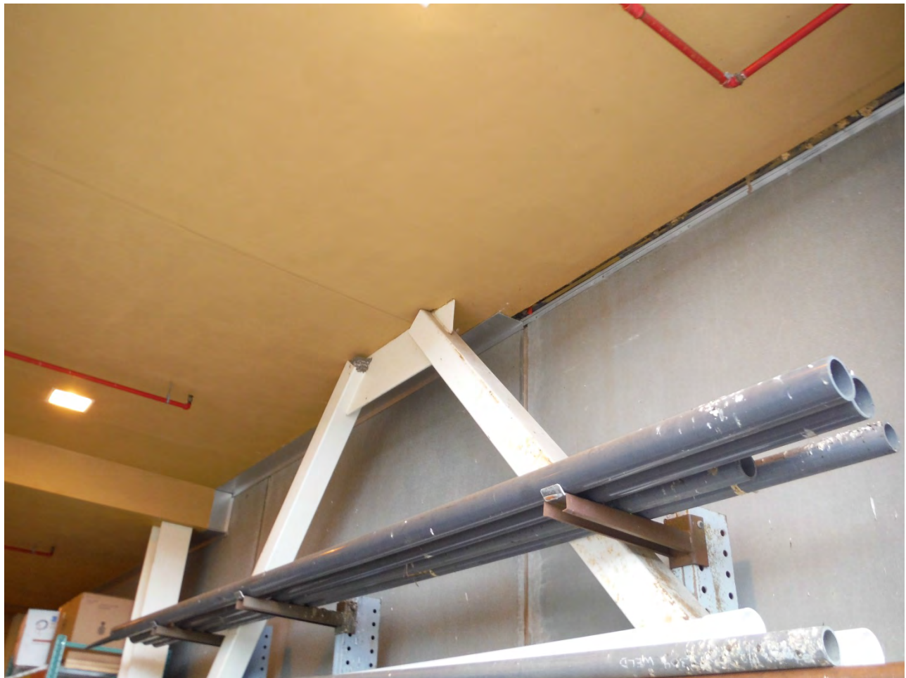
Figure 21. Non-Ductile Detailing of Chevron Braced Frame
