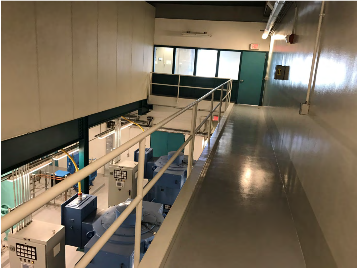
Figure 6. Interior View of Interbay Pump Station
