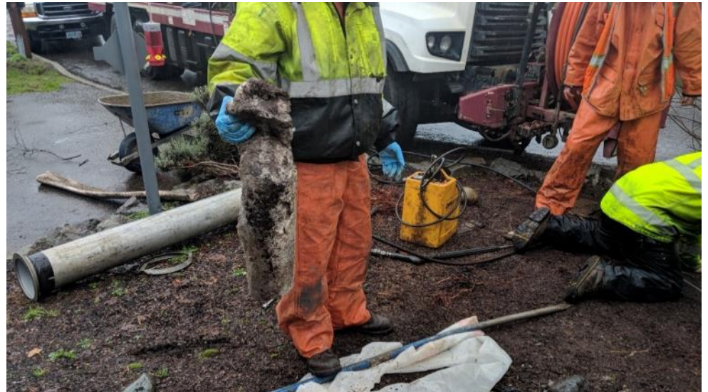
Improperly cured liner portion
