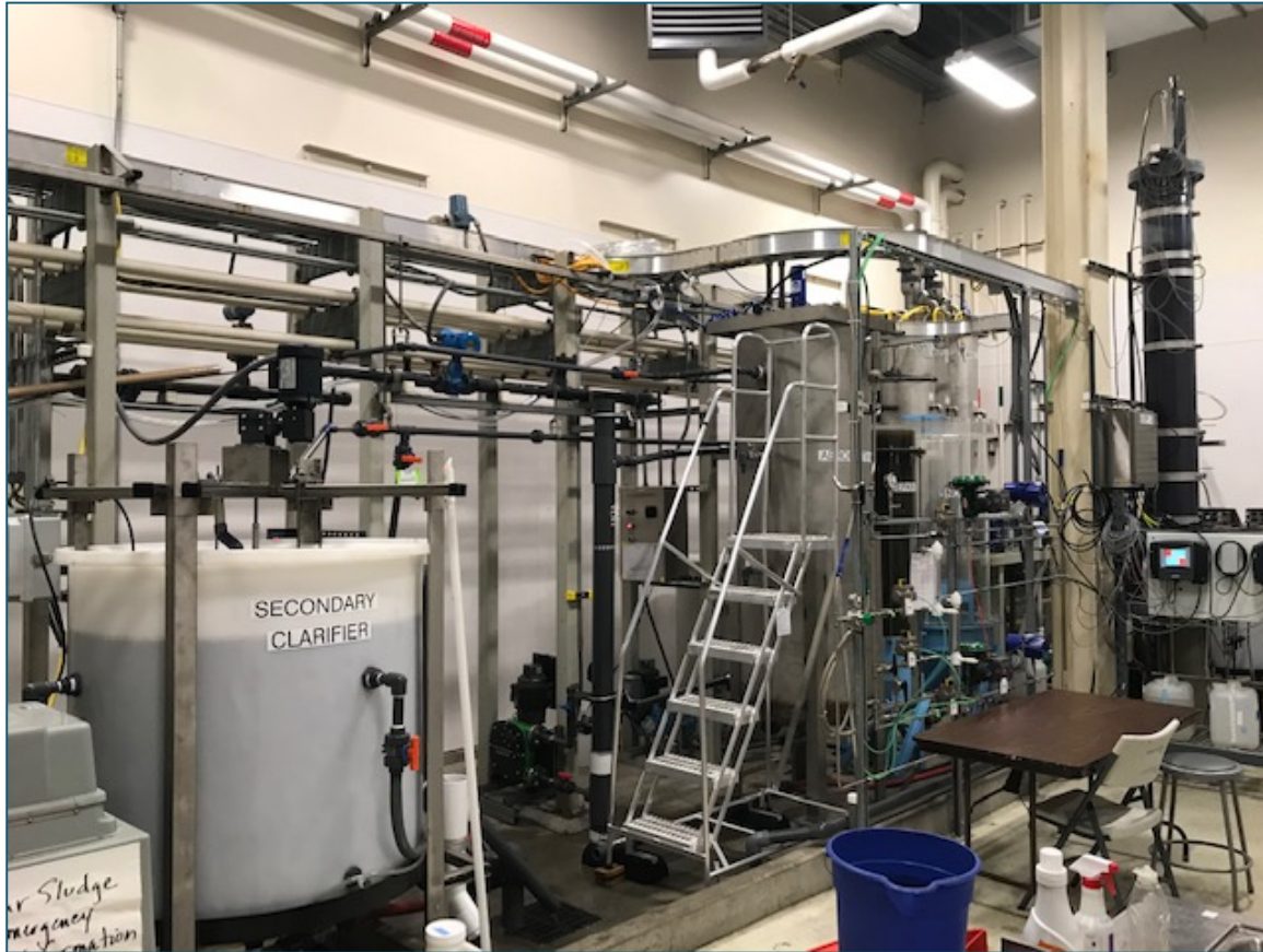
Aerobic Granular Sludge
