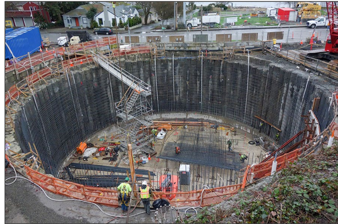
Storage Tank at Murray CSO Control Project
