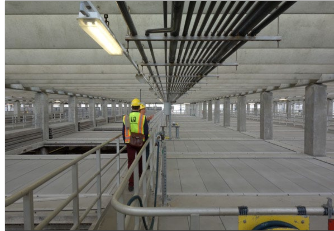
WestPoint Treatment Plant
