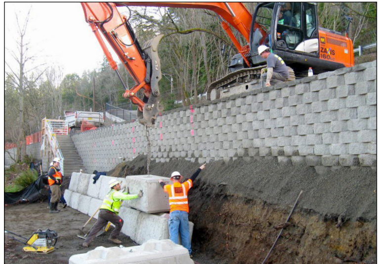
The South Sammamish B segment will include over 50 new walls to support the wider trail and new access stairs, and minimize the trail's footprint.
