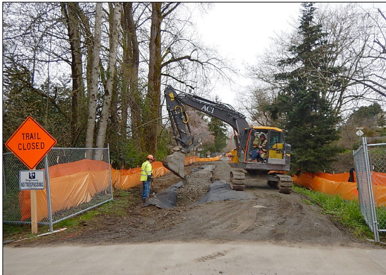
To maintain safety and expedite construction activities, trail sections will be closed during construction.
