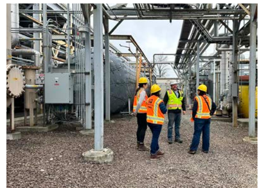
The landfill gas-to-energy plant at Cedar Hills
