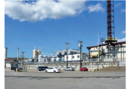
Bio Energy Washington landfill gas-to-energy plant
