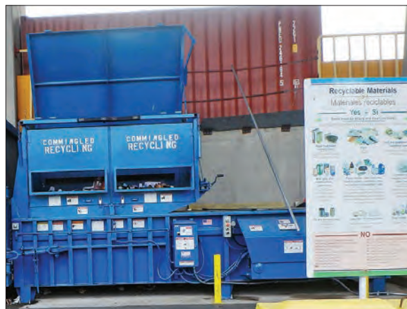
Compactors for recyclable materials
