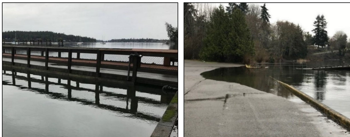
Figure 11. High Tide at Dockton Park During a Storm Event (January 04, 2021), Quartermaster Harbor, Maury Island. (a) Water reached top of bulkhead and bottom of the pier. (b) Dockton Park Boat Ramp is overtopped and water inundates above the ramp bulkhead. Photos: KC (G. Rabourn).
