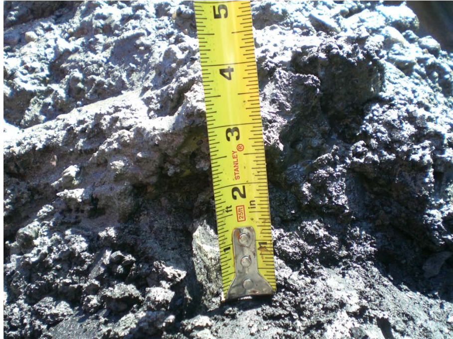
Picture 3-3: Carbonization/Corrosion Layer Shown of Approximately 4" Thickness
