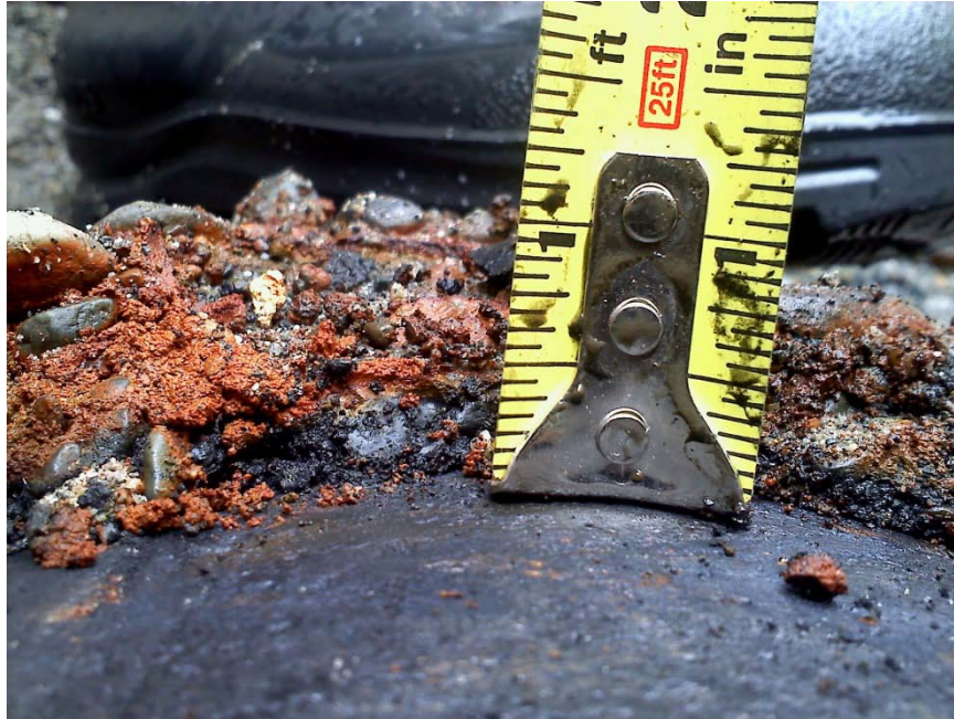
Picture 1-5: Thickness of the Carbonation/Corrosion Product Layer of 1"
