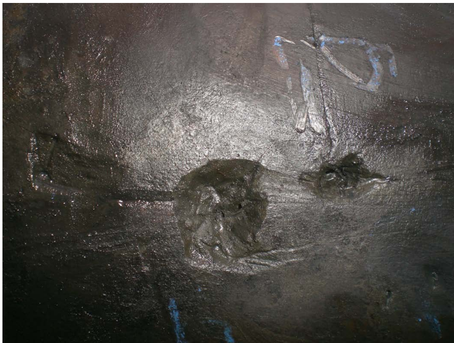
Picture 3-6: Depths of Pits 10 and 11 These pits appeared to be initiated by slight damage most likely from installation.
