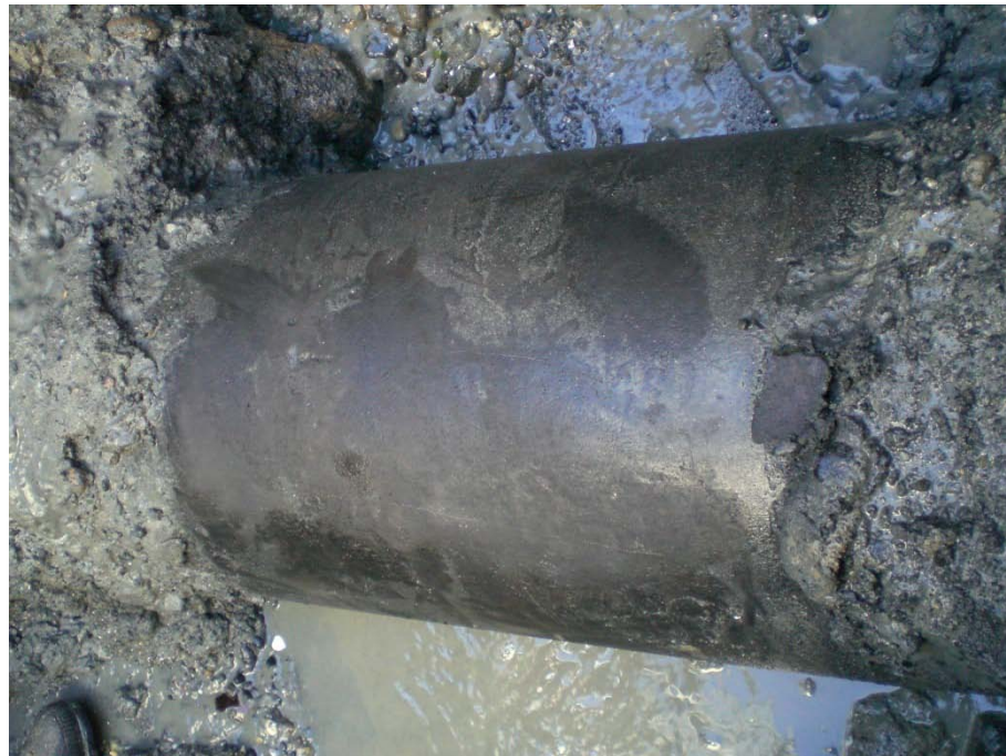
Picture 2-4: General Profile of Pipe with Carbonation Layer Removed
