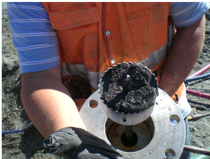
Picture 2-6: Tapping Machine with Coupon Inside & Concrete Lining (This is the only sample that retained the concrete lining.)
