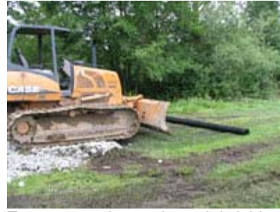
To construct the road, mesh is laid on the surface and rock is spread over the mesh. This temporary road will be removed and the area restored once remediation activity is complete. The University of Washington grounds staff are working closely with King County as work in this area progresses. June 4, 2008
