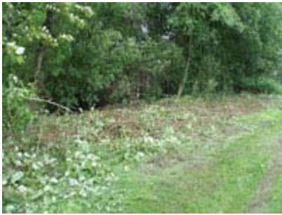
Vegetation by the waterway is being removed to allow access by large equipment. June 4, 2008
