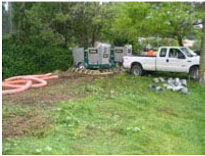
Stormwater flows through the system will be maintained with pumps and bypass pipes to divert water around the cleanup area. June 4, 2008
