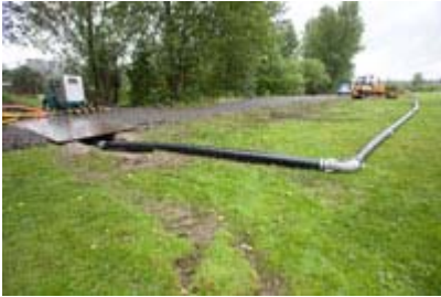
A temporary bypass pipe has been installed to keep incoming stormwater flowing past the cleanup area. June 6, 2008
