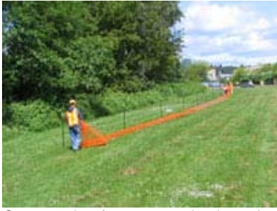
Construction fence extends along the east side of the waterway between 45th and Clark Road. Crews will work inside this area. June 4, 2008
