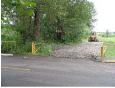
A temporary road is being constructed to allow heavy equipment and trucks into the area. June 4, 2008
