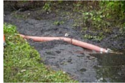
Water was removed from the cleanup area to expose sediments for removal. June 6, 2008
