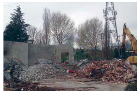
Work includes demolishing aboveground portions of existing buildings like in the example above.
