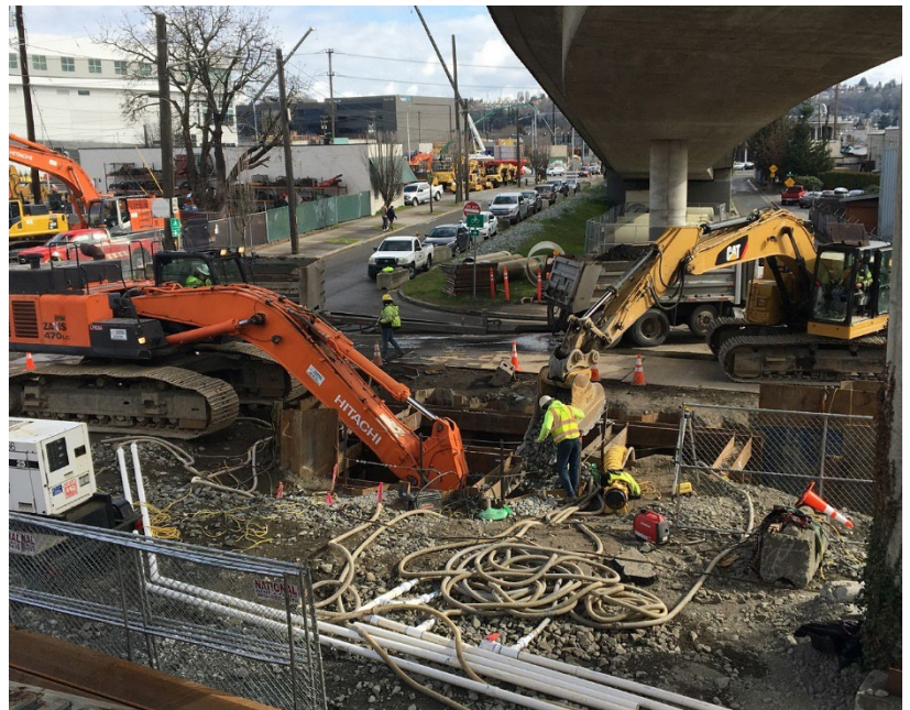
A look down in the trench as it is being prepared for placement of the 60-inch diameter effluent pipe underneath the First Avenue Bridge.
