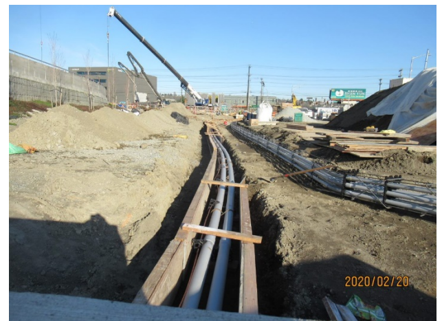
After the duct banks and conduits are installed, they are then back filled and concealed underground.
