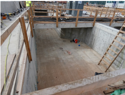
The Treatment Station's UV disinfectant tanks
