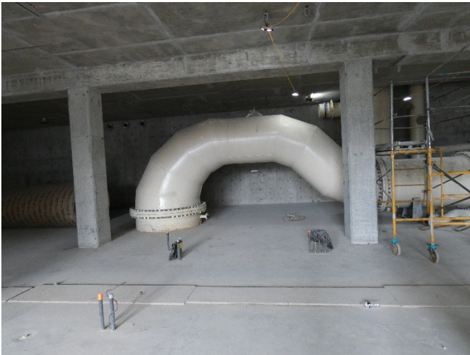
Photo of the interior of the treatment station's ballasted sedimentation building.
