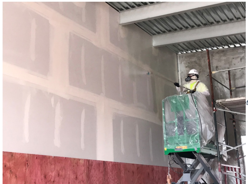
Painting at the treatment station's electrical building
