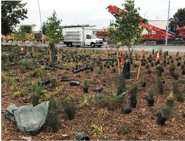
Landscaping and restoration work between East Marginal Way and the SR-99 onramp.
