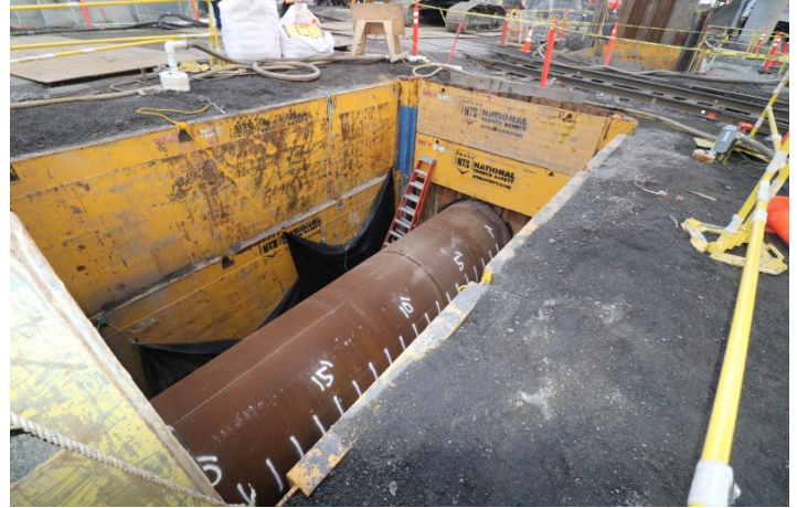
72-inch steel casing pipe underneath the First Avenue Bridge near the intersection of South River Street and South Michigan Street.
