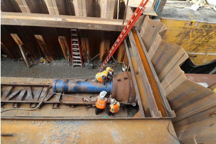
Crew install pipes using a “pneumatic” or air powered hammer to drive steel casing pipes into place at the conveyance site.
