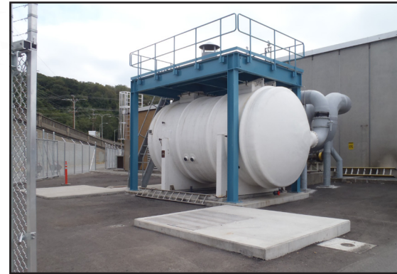
Carbon scrubber at Interbay Pump Station.
