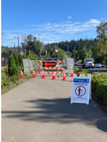
Caption: Dismount sign for cyclists on the pedestrian pathway next to 120th Avenue Northeast to safely pass through the construction detour.
