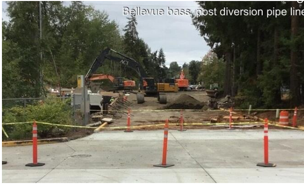
Caption: Restoration of excavated surfaces for the temporary diversion pipe are in progress at 124 th Ave NE.
