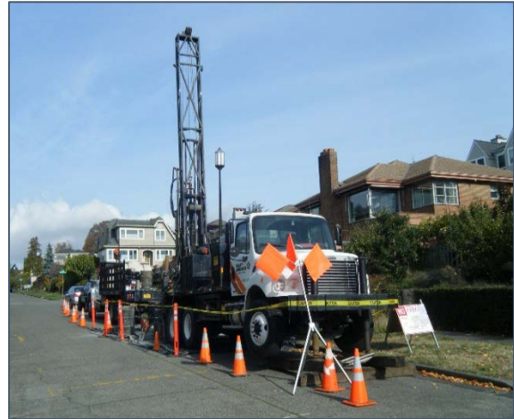
Crews will use a truck-mounted drill rig to take soil samples along the roadway.
