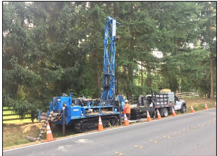
Crews will use a track rig to take soil samples at 180th Avenue N.E. and N.E. 30th Street.
