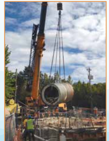
The microtunneling machine will be placed into the shaft using a large crane.
