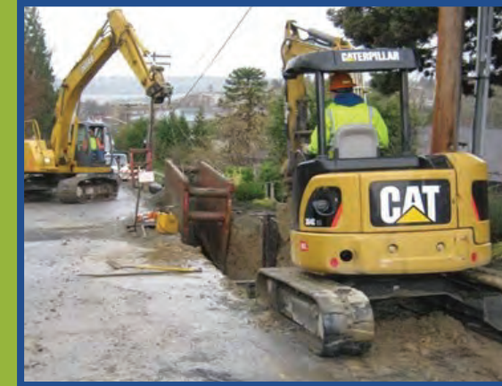
An example of King County crews excavating before installing a sewer pipe under a roadway.
