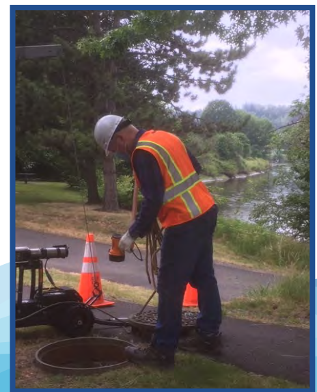
You may see King County crews out inspecting sewer pipes in your neighborhood. Their work is essential to protecting public health and keeping our waters clean.
