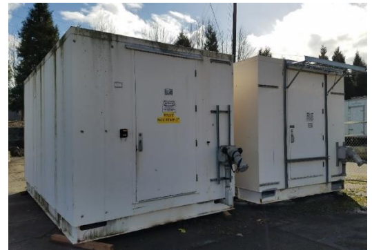
Trailers like these may house generators or other controls for the temporary pump station.
