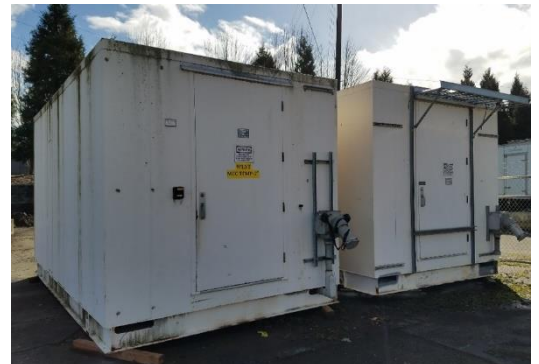
Trailers like these may house electrical equipment or other controls for the temporary
