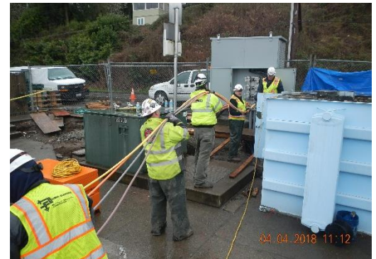
An example of what electrical work at the pump station might look like.
