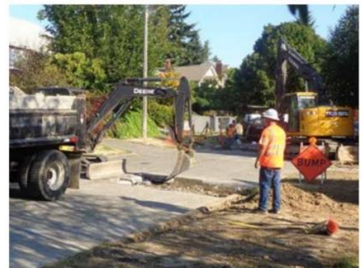
Example of traffic control personnel and what roadway work may look like.
