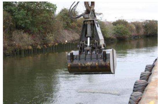
An example of equipment that is used to remove soil from a lakebed
