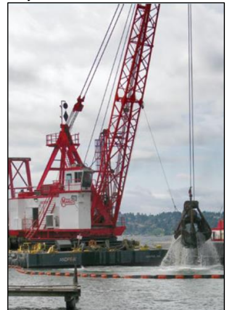
A barge-mounted crane uses a clamshell to remove materials from the lakebed.
