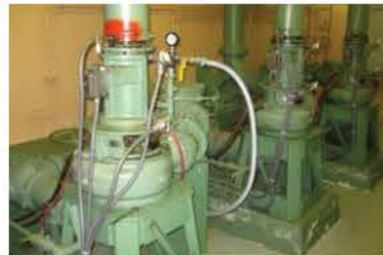
Pumps will be upgraded at the North Mercer Pump Station
