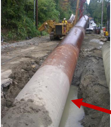
48-inch Conductor Casing
