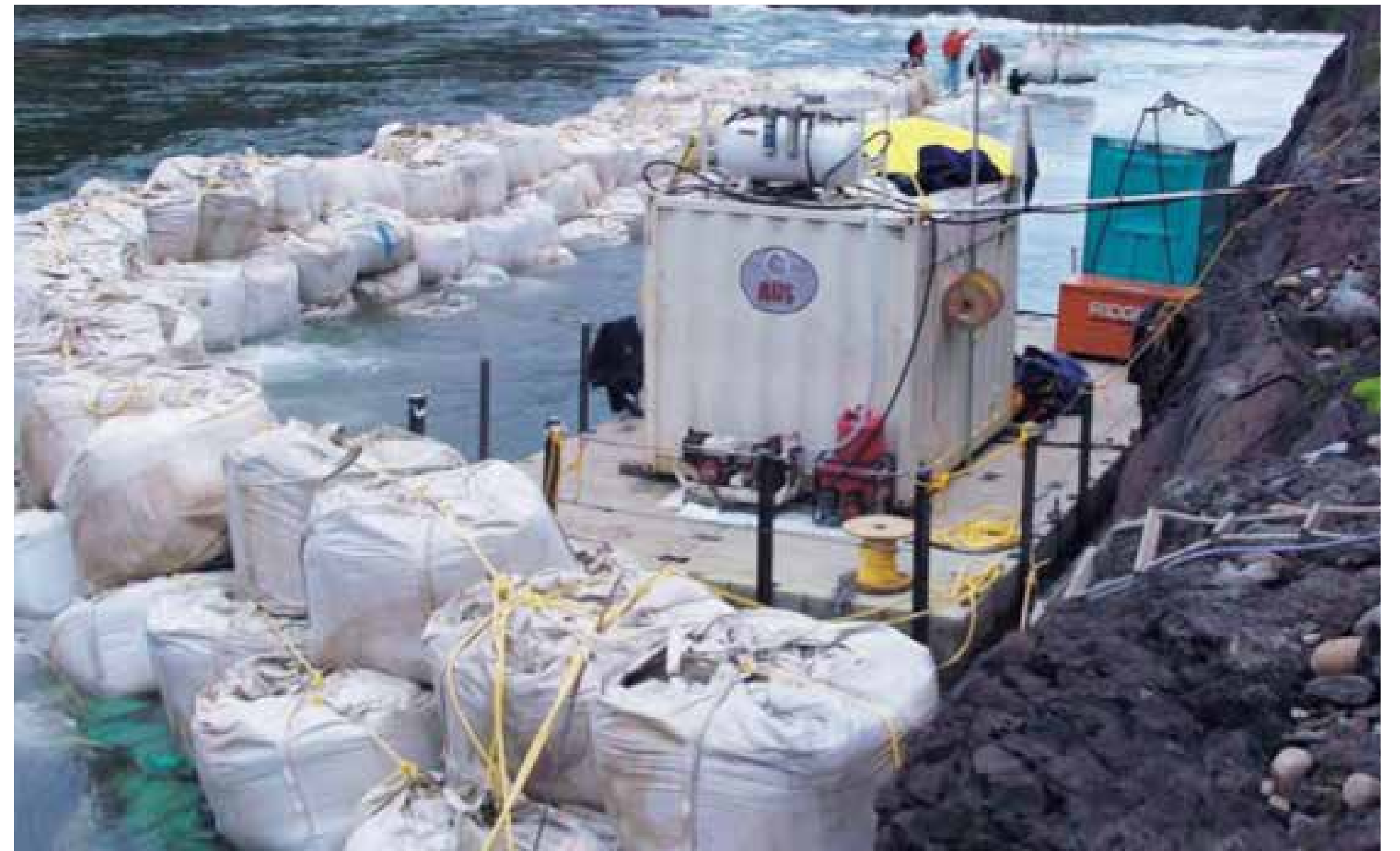
Construction work at Enatai Beach Park and Mercer Slough will be contained within what are known as dry cells that protect habitat and water quality outside of the construction zone.
