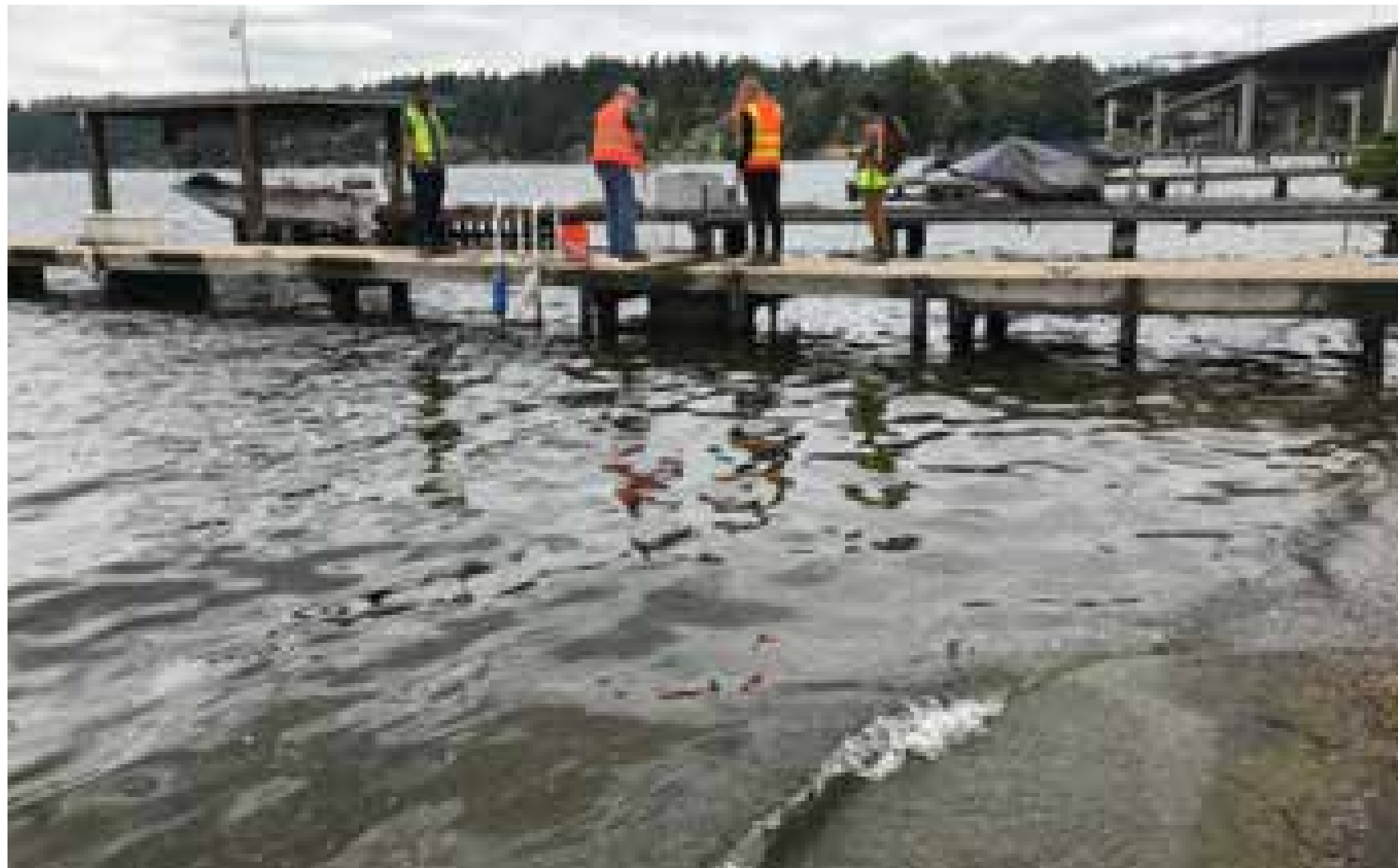
The existing pipeline will be accessed from the various maintenance holes that run along the line from Enatai Beach Park, under some docks, and up the Mercer Slough.
