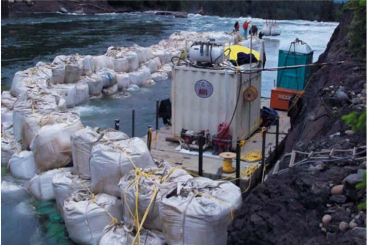
Construction work at Enatai Beach Park and in Mercer Slough will be contained by "super sacks" that protect habitat and water quality outside of the construction zone.
