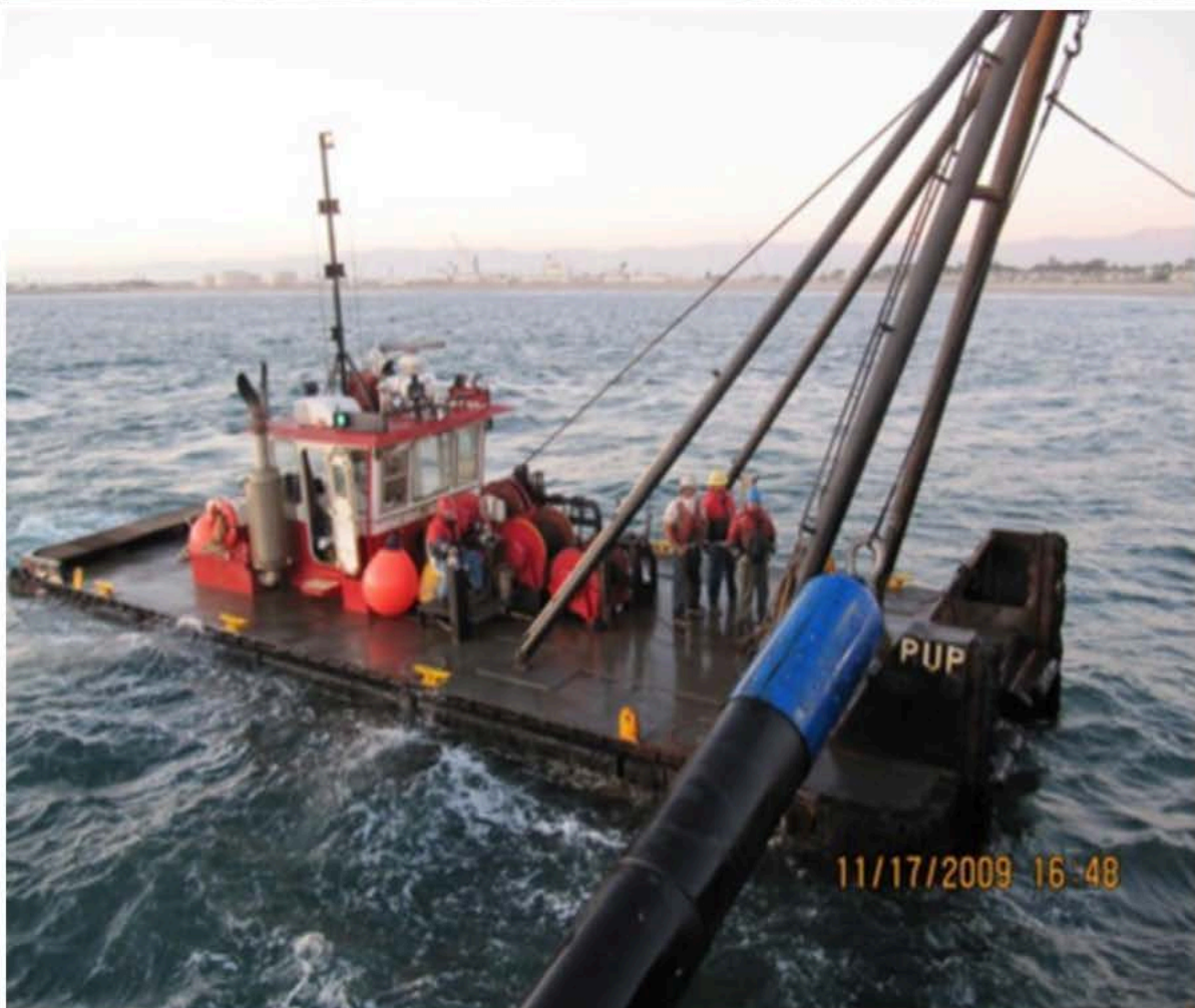
Most of the repair work will take place from barges in the water. The barges will be moved throughout work progress.
