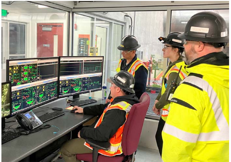
A King County operator shows operators in training and a safety officer what's happening in the Brightwater treatment system.
