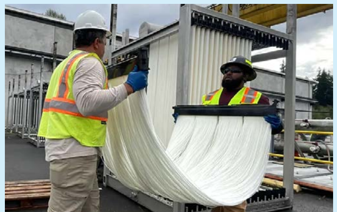
A King County utility worker and a contractor work together to install new membrane filters.
