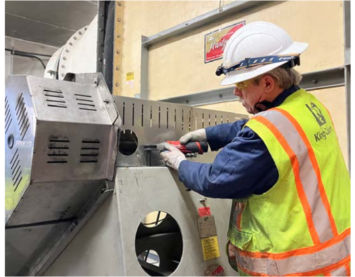
A King County mechanic maintains odor control equipment at Brightwater.
