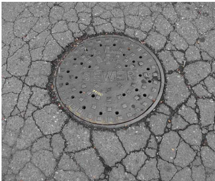
Manhole with indications of settlement in the pavement that likely subject the cover to inundation during rainfall. The large number of pick holes in the lid also allows free flow of surface water into the manhole.
