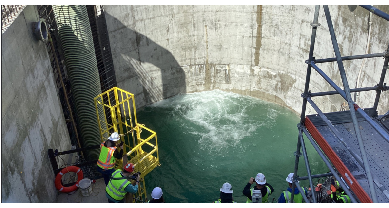
The Ship Canal Water Quality Project is a joint effort between King County and Seattle Public Utilities. The project will capture and store 29 million gallons of polluted water during heavy rains. An underground storage tunnel is being built to hold the stormwater and sewage until there is room to send it to the West Point Treatment Plant. It will control four CSO outfalls for the City of Seattle and two King County outfalls at 3rd Ave W and 11th Ave NW. Construction is ongoing.
