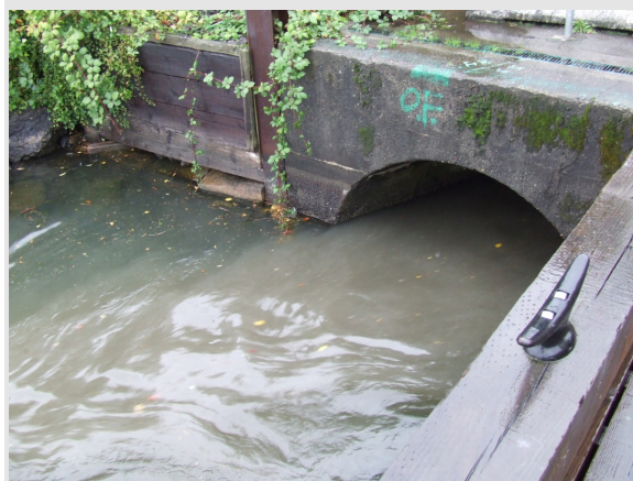
University Regulator Station Overflowing 10/26/09
