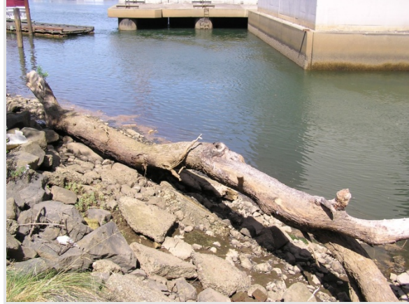
West Michigan Regulator Station CSO Vicinity; Looking North at the First Avenue South Bridge Footing
