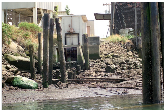
Brandon Street Regulator Station CSO Overflow at Extreme Low Tide
