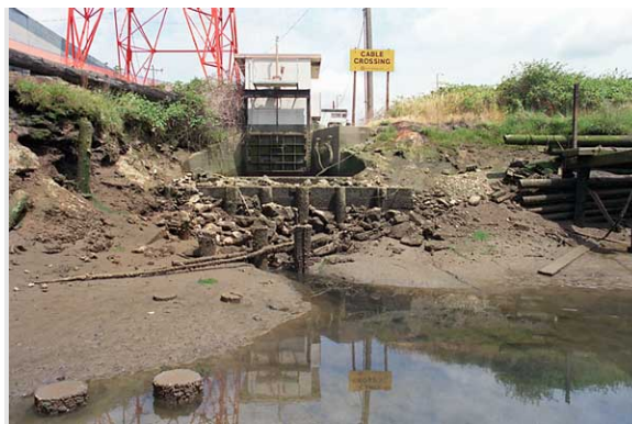
South Michigan Street Regulator Station CSO at Extreme Low Tide
