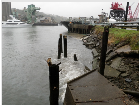
Brandon Street Regulator Station CSO Overflowing 10/17/09
