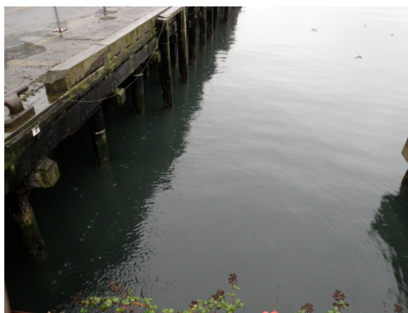
King Street Regulator CSO Overflowing 10/26/09
