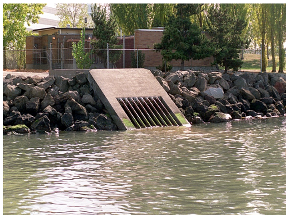
Denny Way Original Outfall
