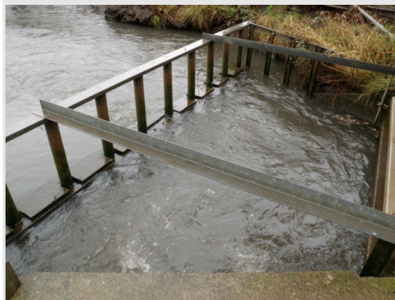
South Michigan Street Regulator Station CSO Overflowing 10/26/09
