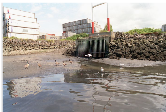
Diagonal Storm Drain (Hanford #1) Outfall at Low Tide; Grate Is Now Gone.
