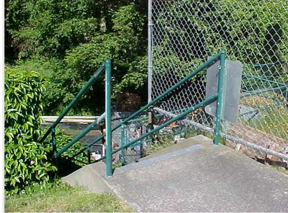
30th Avenue Northeast and Belvoir Place Pump Stations' CSO Vicinity; Looking Southwest, No Warning Signage Because No Public Access
