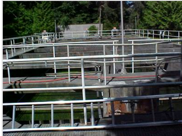
Carkeek Wet Weather Treatment Station Sedimentation Tanks
