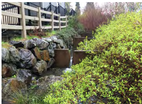
Top left: rain garden Top right: bioretention in Ballard Bottom left: cistern installation Bottom right: cascading bioretention in Broadview
