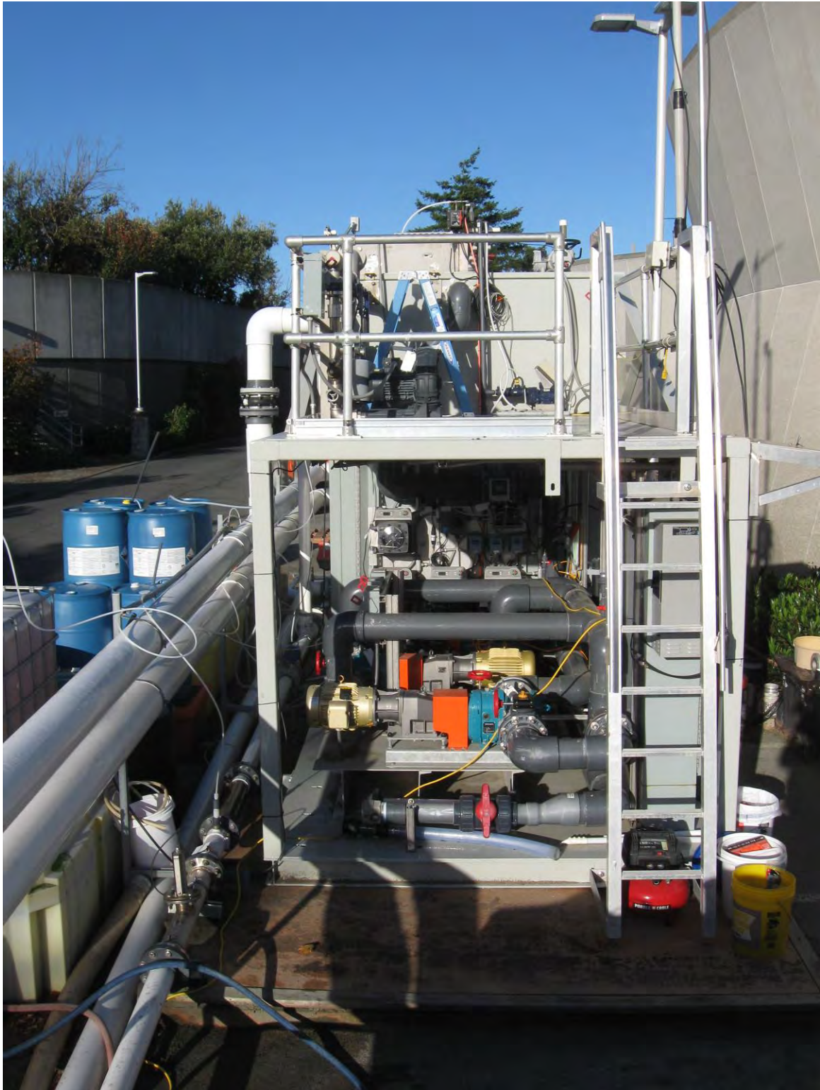
Figure 1-5. Pilot Unit Equipment Area, with Permeate/Backwash Pumps (bottom front), Chemical Feed Pumps (back wall), PLC (cabinet behind ladder), and Blowers (upper)
