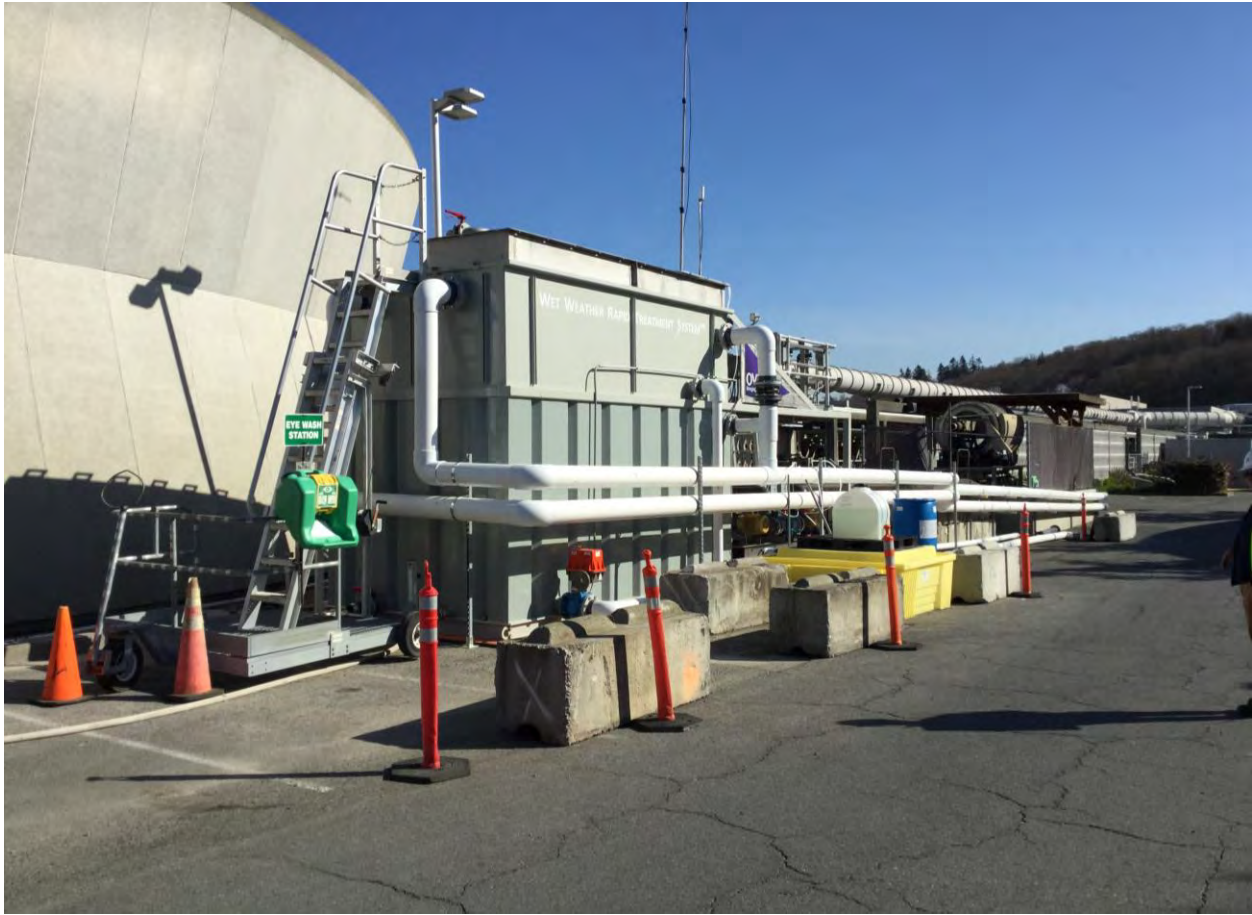
Figure 1-3. Permeate Tank Overflow Pipe (behind staircase) and Membrane Tank Overflow Pipe (right of staircase)
