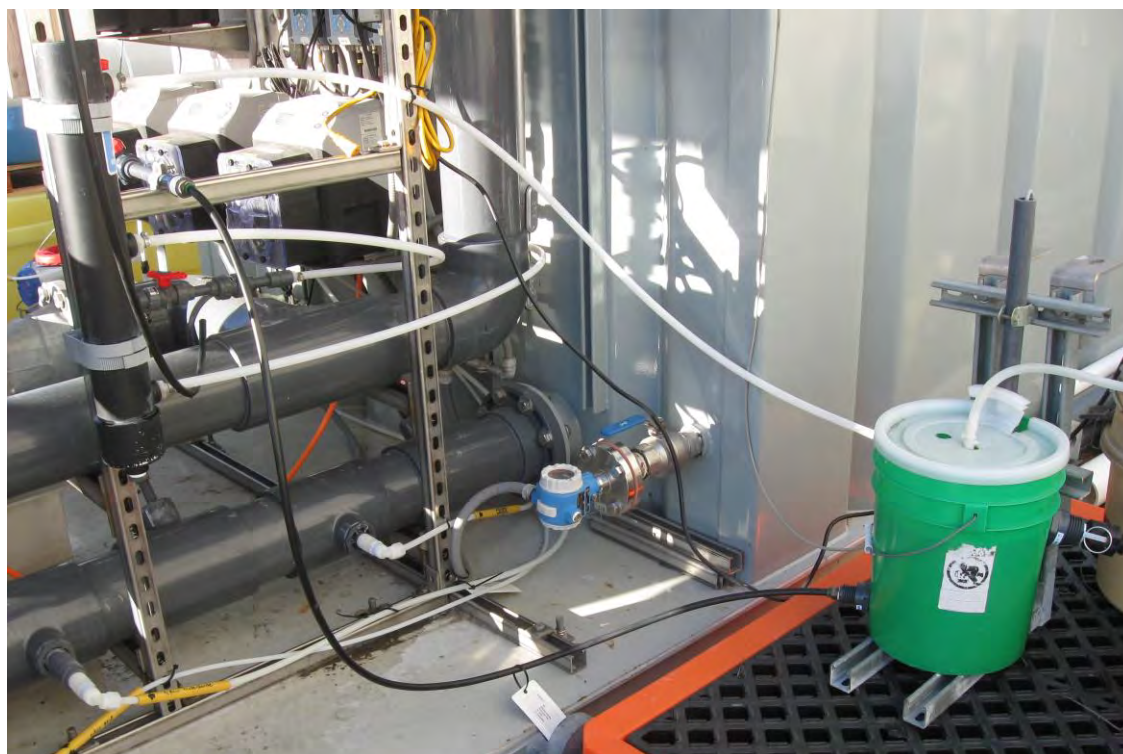
Figure 1-6. Effluent Sample Line and Sample Bucket
