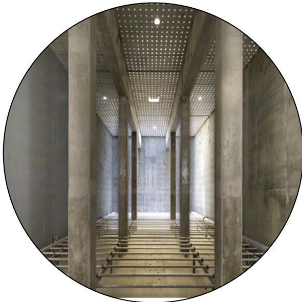
Interior of BIOSTYR Cell
