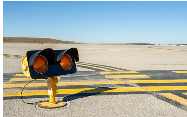
Elevated Runway Guard Light
