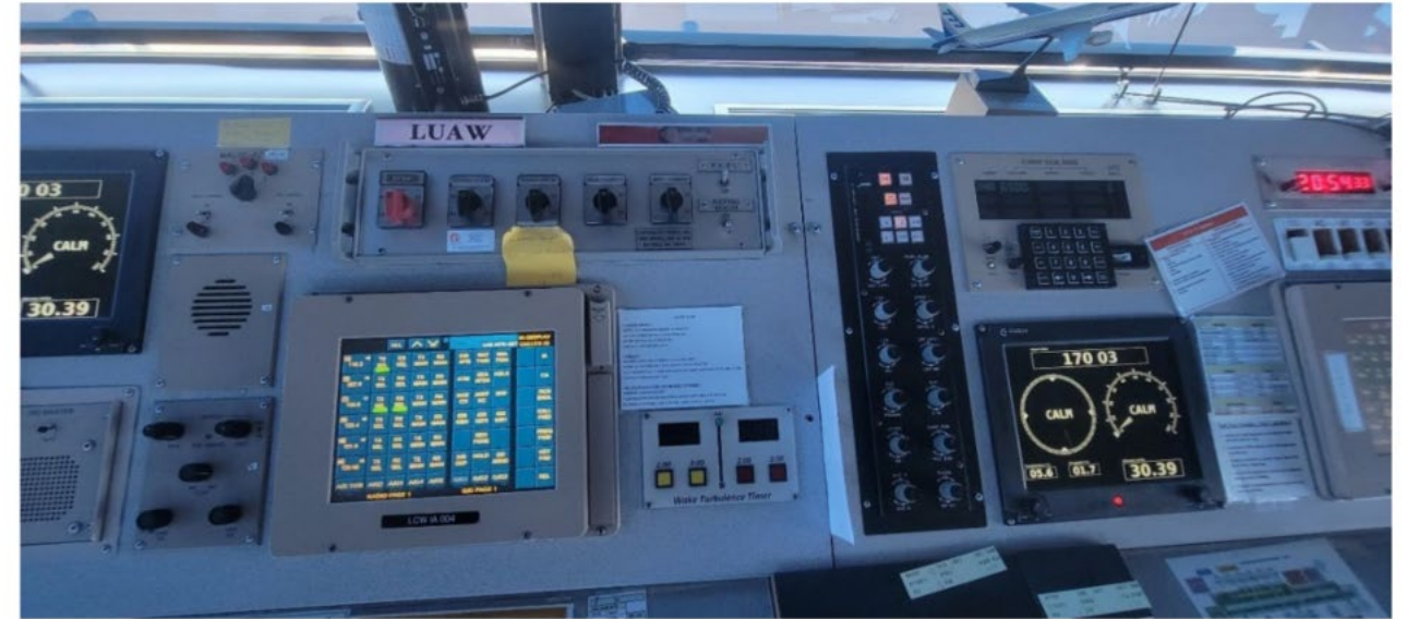
ATCT CAB, Existing CCR Control Switches
