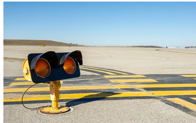
Elevated Runway Guard Light
