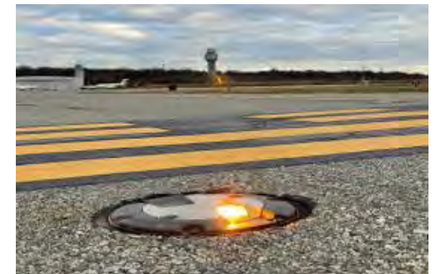
In-pavement Runway Guard Light
