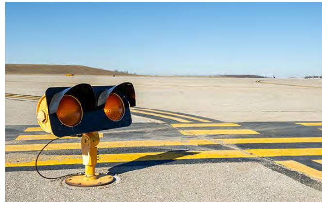
Elevated Runway Guard Light
