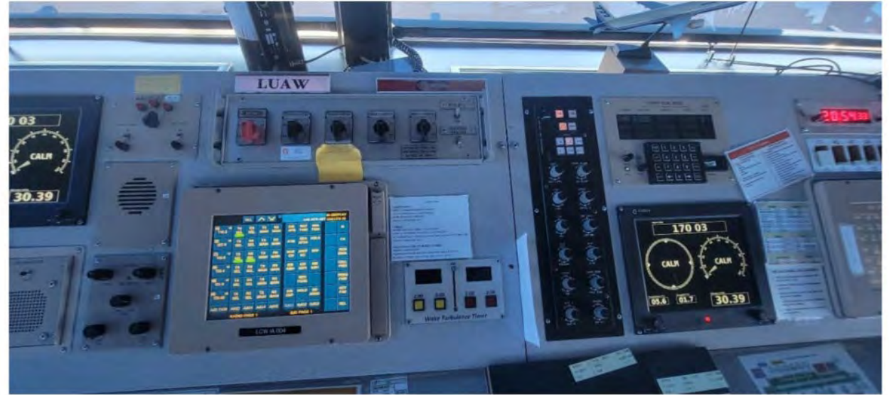
ATCT CAB, Existing CCR Control Switches
