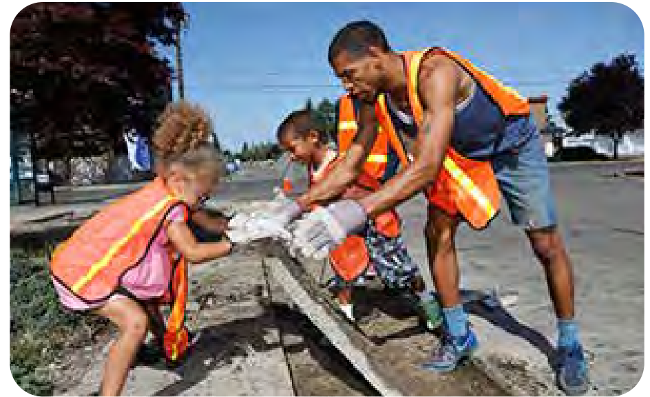
Figure 25. McKinley Hill Neighborhood depaving project, Tacoma, Washington. Photo source: Pierce Conservation District .
