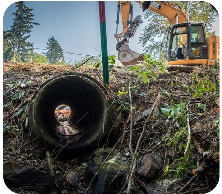
Replacing culverts that block access to high quality stream habitat is important to helping salmon survive and thrive in a changing climate.
