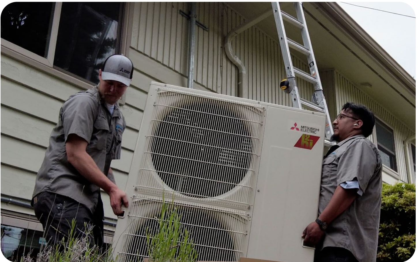
King County's Energize Heat Pump Program installs heat pumps and other clean technology to help low and moderate-income homes in King County.
