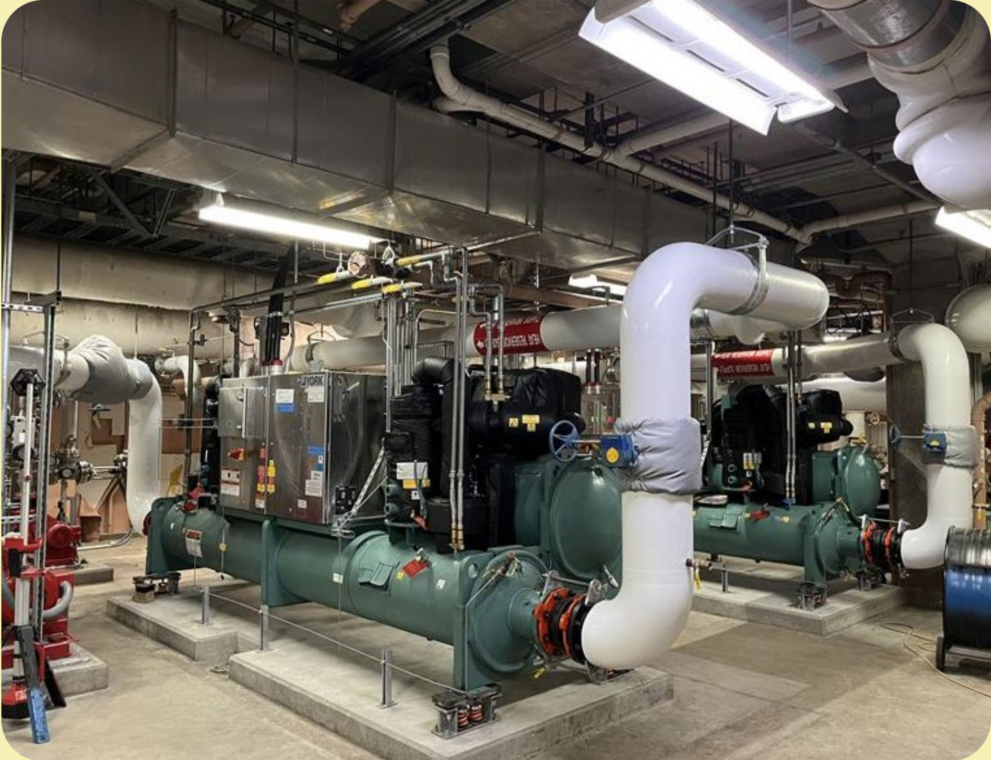
New industrial heat pumps at the South Wastewater Treatment Plant are significantly reducing natural gas usage.
