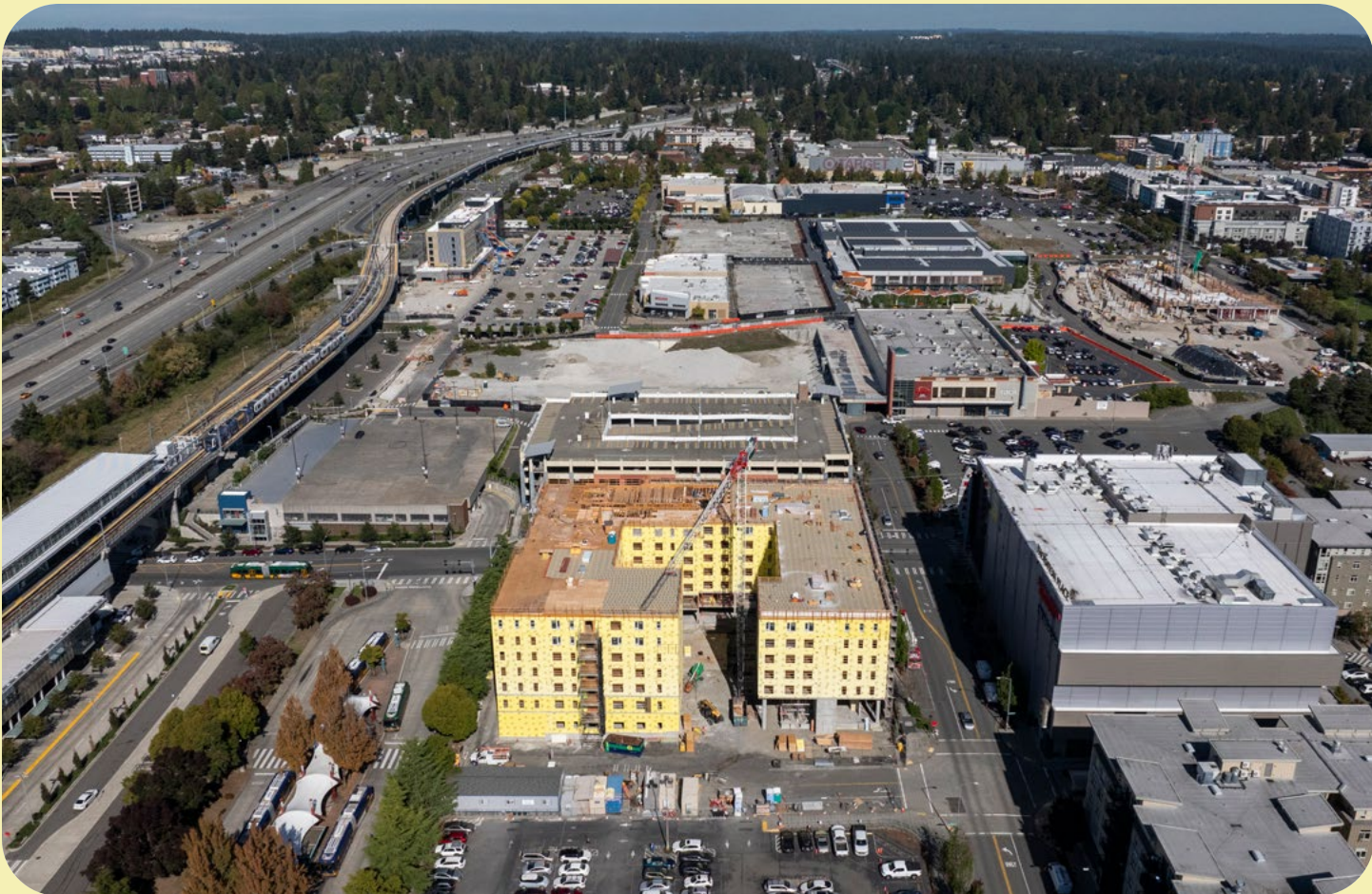
Transit Oriented Development under construction at Northgate Light Rail Station – BRIDGE Housing and Community Roots Housing.
